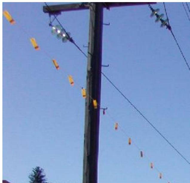
Figure 6: Example of visual tape bunting fitted under overhead power lines.
